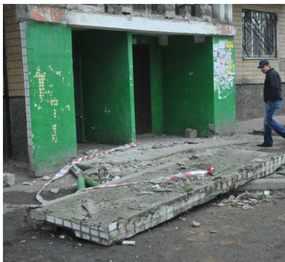
Fig. 2. Collapse of the cantilever slab of the covering of the entrance group
