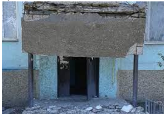
Figure 1. Failure of the cornice slab above the entrance to the building.
