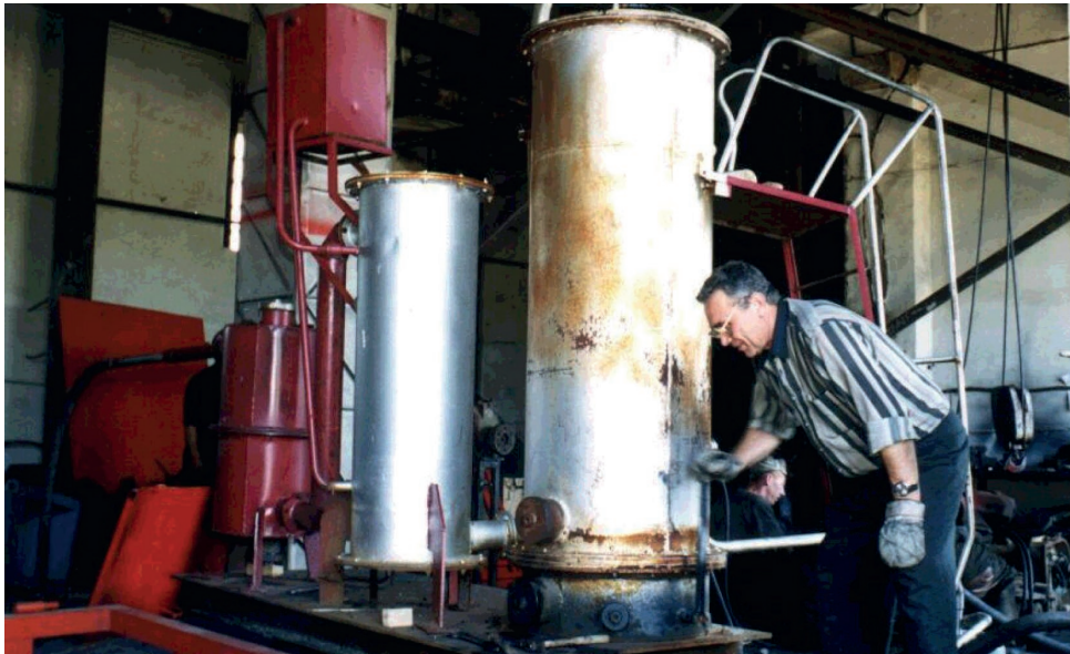
Figure 5. General view of the gas generator GG-30
